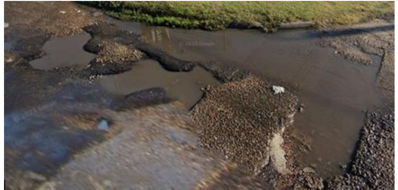
Pothole filled with water on Francia Street
