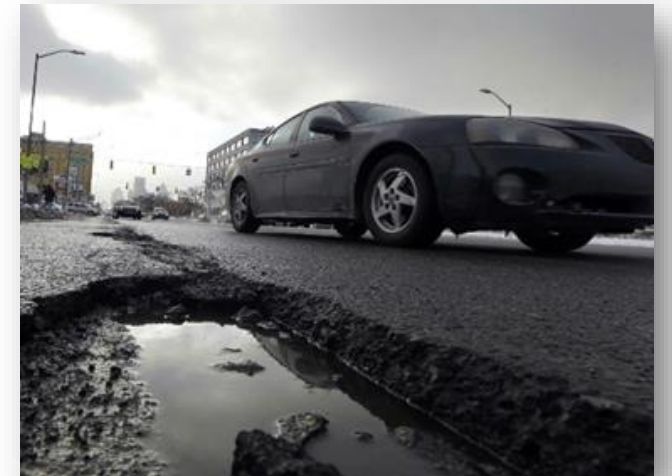
Vehicle's safety hazard because of this pothole
