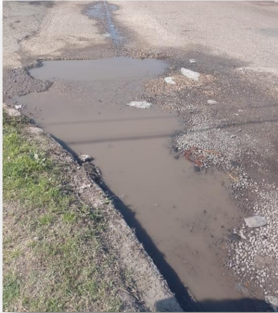
Pothole at the intersection of Rio Negro Street and Francia Street
