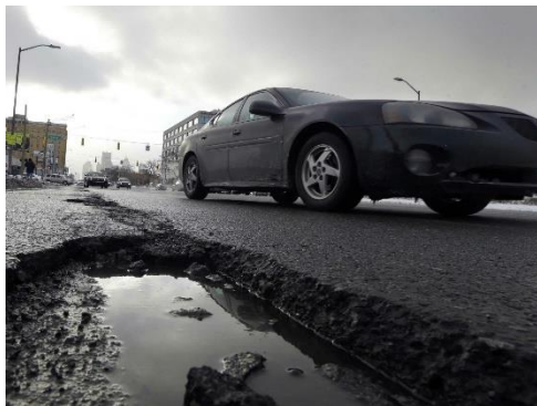
Fig. 13. Vehicle's Safety Hazard because of this pothole.
