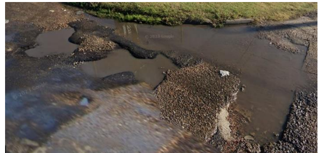
Fig. 5. Pothole filled with water on Francia Street.
