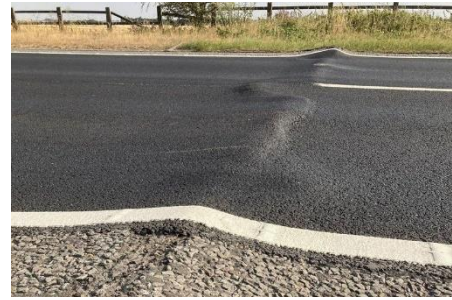
Fig. 8. Impact of extremely high temperature on pavement quality.
