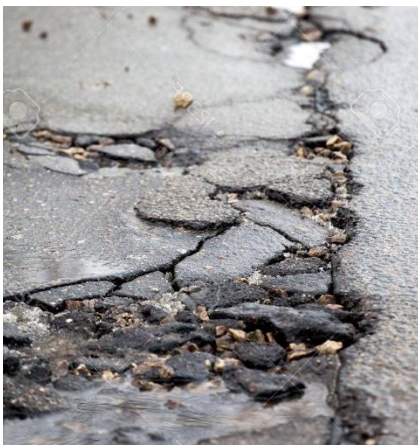
Fig. 7. Impact of extremely low temperature on pavement quality.
