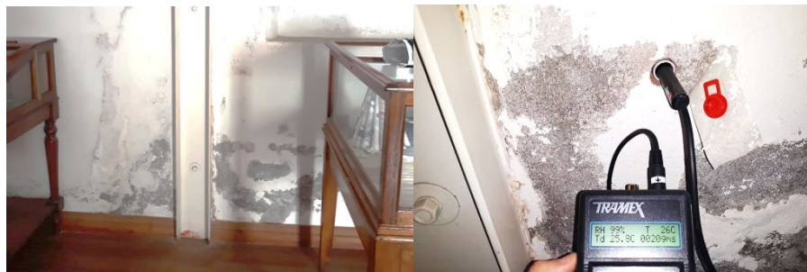
Fig. 8 Provision of probes to measure internal wall moisture and measurement (a). Internal humidity measuring point in room 3 (b)
