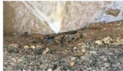
Corrosion pin hole on an iron pipe.
