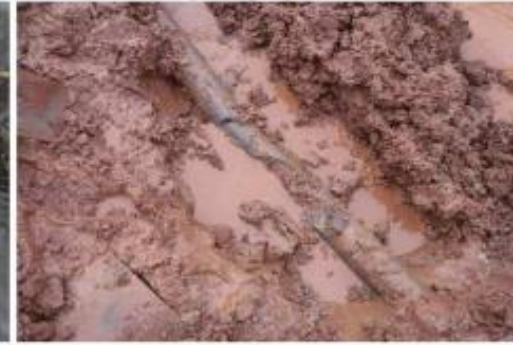
Longitudinal split on a polyvinyl chloride pipe.
