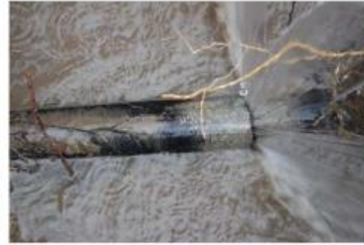
Circumferential break on an asbestos cement pipe.
