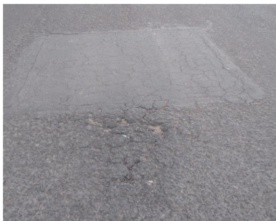
Fig.14. Roadway deterioration and repairs.
