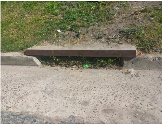
Fig. 10. View of a clogged storm drain.
