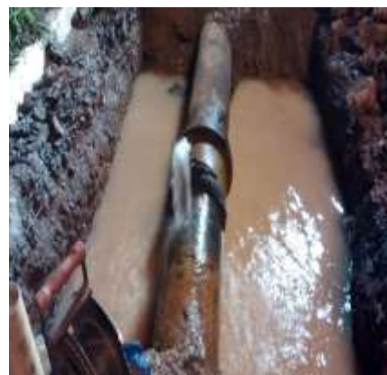
Fig. 2 Rupture of a mother pipe in the city of Concordia, Entre Rios, Argentina in 2016 [11]
