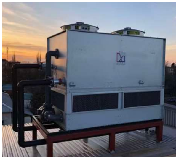
Ilustración 4.29. Torre de enfriamiento. Fuente: https://sxstwt.en.made-in-china.com/product/HQspVOwCrucG/China-15m3-H-Well-Borehole-River-Lake-etc-Reverse-Osmosis-Water-Purification-Plant-RO-Water-Purifier-for-Drinking.html?pv_id=1iv31boc1d13&fav_id=1iv31cgpbea7&bv_id=
