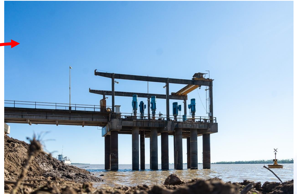
Water extraction pump
