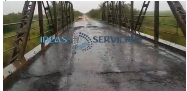
Fig. 5. Damaged surface of the bridge in Paso Bravo, Feliciano.
