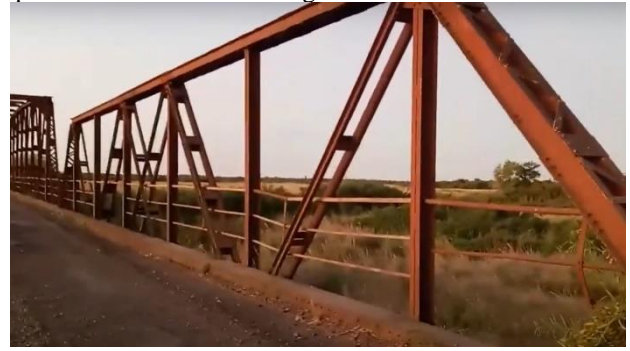
Fig. 4. Bridge in Paso Bravo Feliciano with visible rust and wear.
