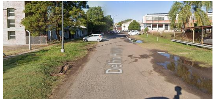
Fig. 5. Potholes with water.
