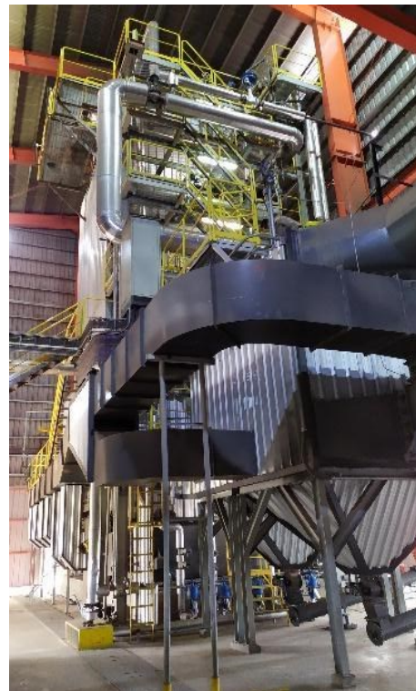
Figura N°1.8: Caldera Acuotubular (22000 kgv/h x 45 bar x 120 °C).
