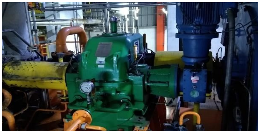
Figura N°1.14: Turbina (Marca TGM-TMC5000/RTS400).
