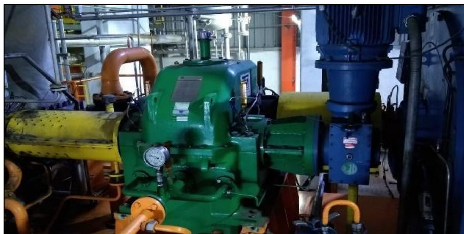
Figura N°1.14: Turbina (Marca TGM-TMC5000/RTS400).
