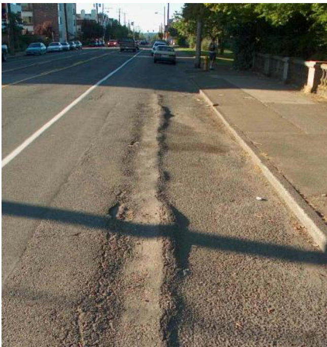
Fig. 4. Example of rutting in a flexible pavement [11].
