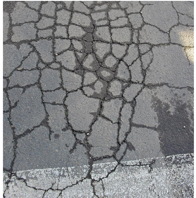
Fig. 5. Example of fatigue cracking in a flexible pavement [12].
