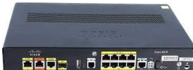
Figura 5. 4 - Router Cisco 891F
