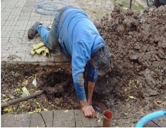
Fig. 3. A broken pipe.
