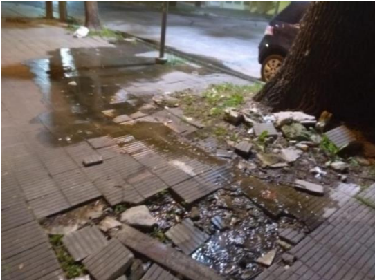
Fig. 4. Water gushing onto the sidewalks.
