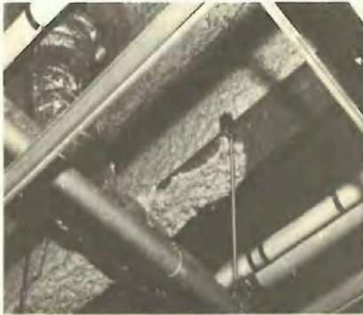
Area Above Suspended Ceiling With Friable Material
