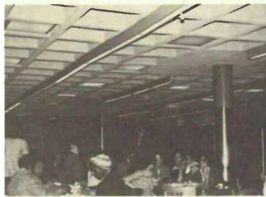
Cafeteria With Friable Material Ceiling Surface
